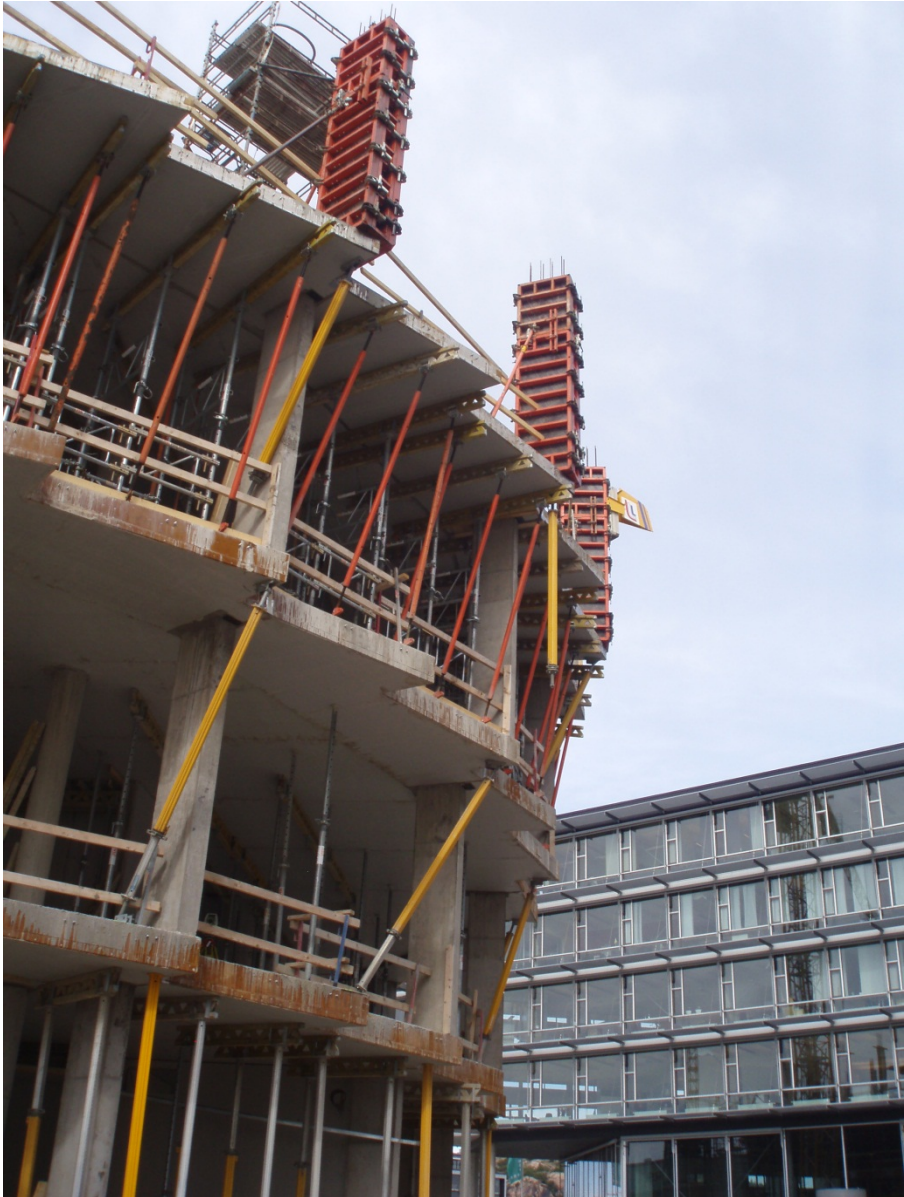
Figure 4 Column formwork on the third floor, shoring towers and slab props hanging from the overhanging pre-cast concrete formwork elements on the second floor, slab props attached to the floor structure below on the first floor and formwork girders, shoring and slab props on the entrance floor.
